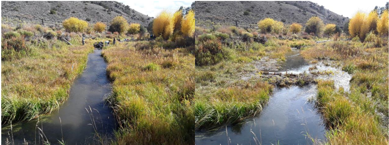
Figure 10. The Kremmling Field Office (CO) installed 60 beaver dam analogs and other LTPBR structures in Reeder Creek in September 2021 to mimic, promote, and sustain beavers and the natural processes that this keystone species performs in healthy riverscapes. This work expands on decades of riparian improvement brought about by managed grazing. The project brought together private practitioners, staff from several BLM offices, and other NGO partners to work on the treatments while learning about the benefits of LTPBR and beaver restoration. The photos were taken before and immediately after treatment. Photo credit: Mark Beardsley, EcoMetrics.
