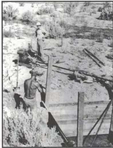
Above: Howard Kimmerle standing by the pump (center of photo). Man in foreground is probably John Kimmerle, who looks like he is tamping the dirt around the form.
