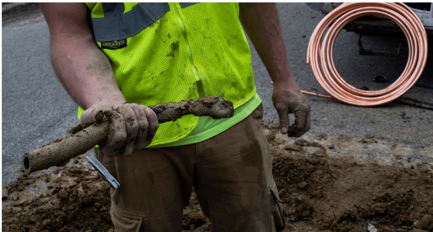
A piece of lead pipe removed during a service line replacement in Flint, Michigan.
