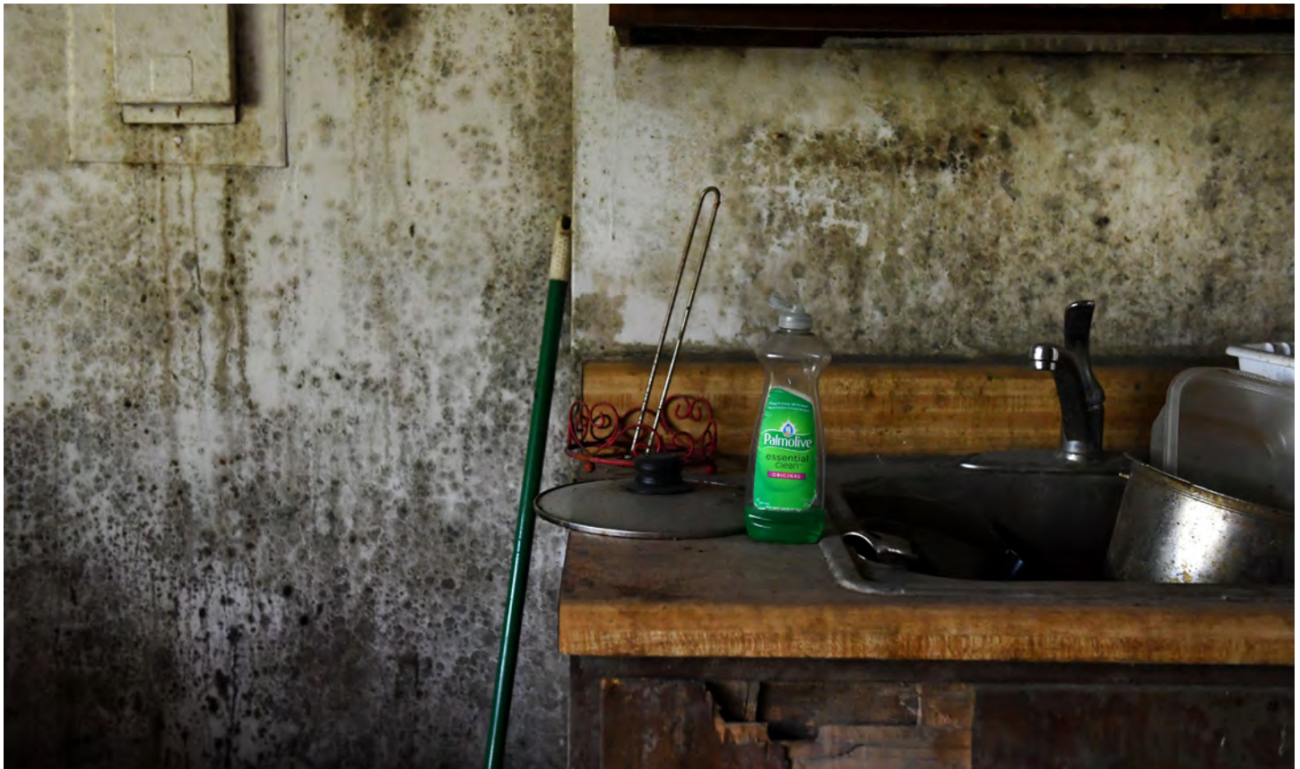
Flooding, leaks, and other sources of excess moisture can promote harmful mold growth indoors.
