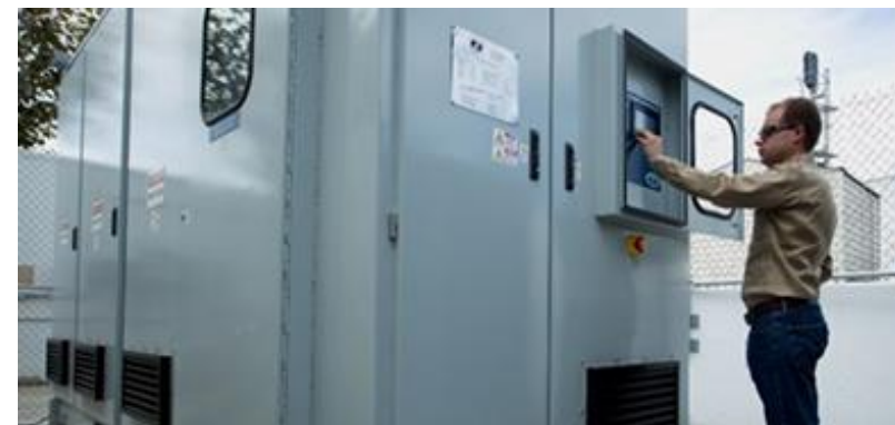
Building Energy Storage Systems Source: https://www.sce.com/safety/bess
