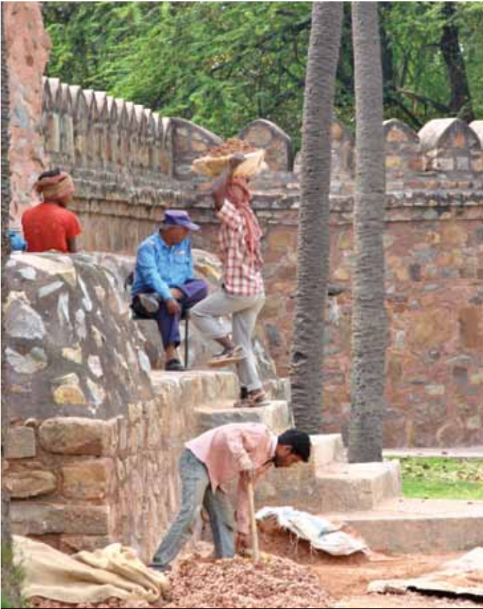
Construction workers exposed to direct sun at noon, March 2012.
