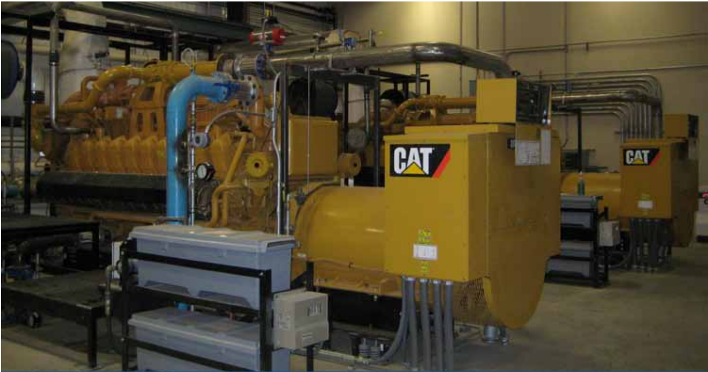
Reciprocating engine prime mover.
