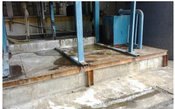
Holding tank for condensate recovery
