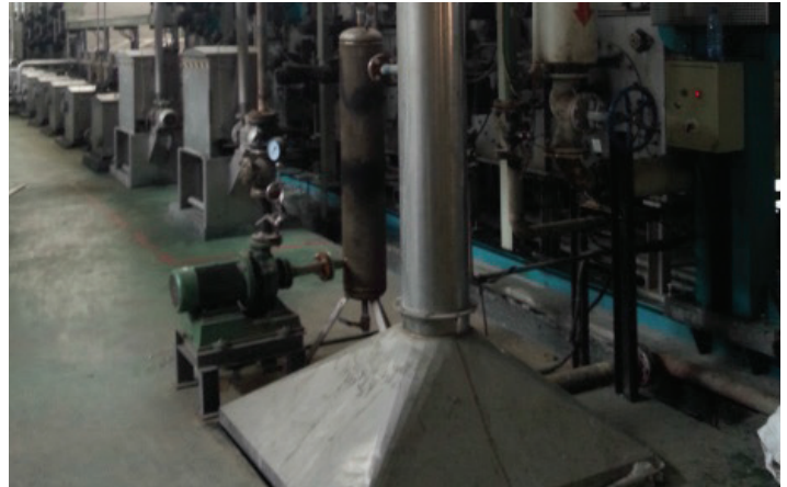
Condensate water recovery
