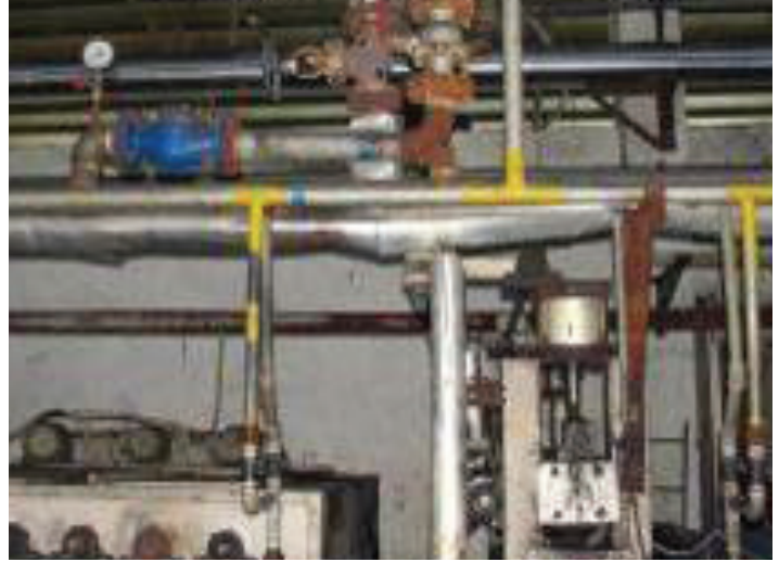
Cooling water recovery pipes system
