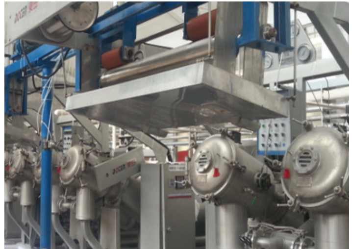
Water squeeze and recovery system
