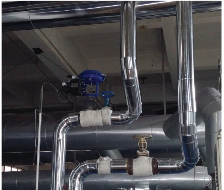
Metering and control system
