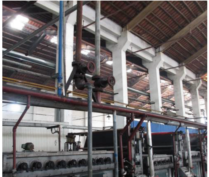
Installed water meters
