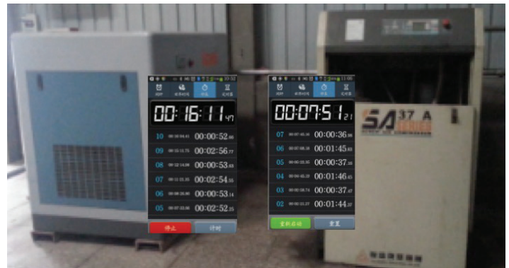
Compressed air leakage detecting and optimizing
