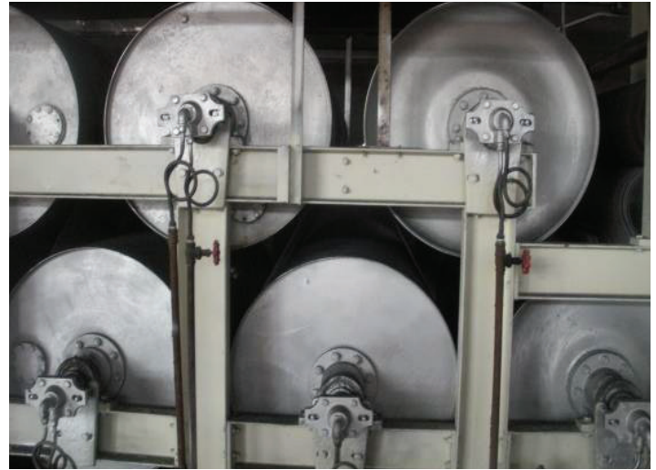
Drying cylinders with insulation on side face
