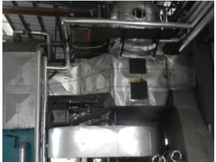
Waste heat boiler
