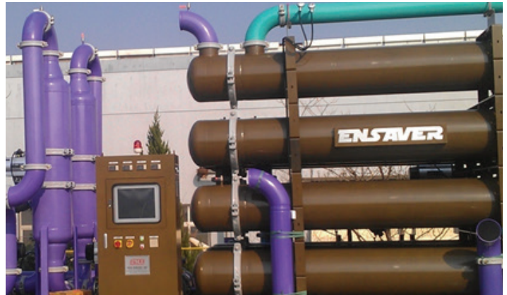
Centralized high efficiency waste water heat recovery system
