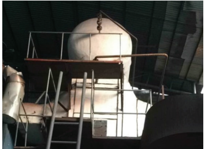
Insulation on Waste Heat Boiler
