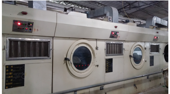
Heat recovery from drying machines
