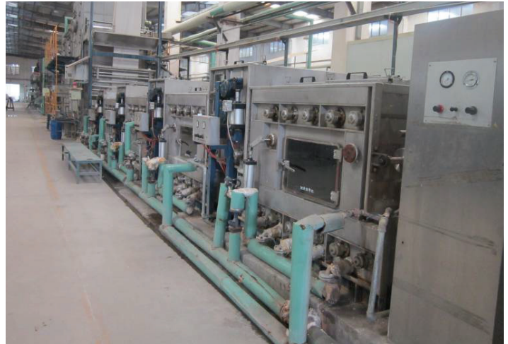
Counter current rinsing retrofit
