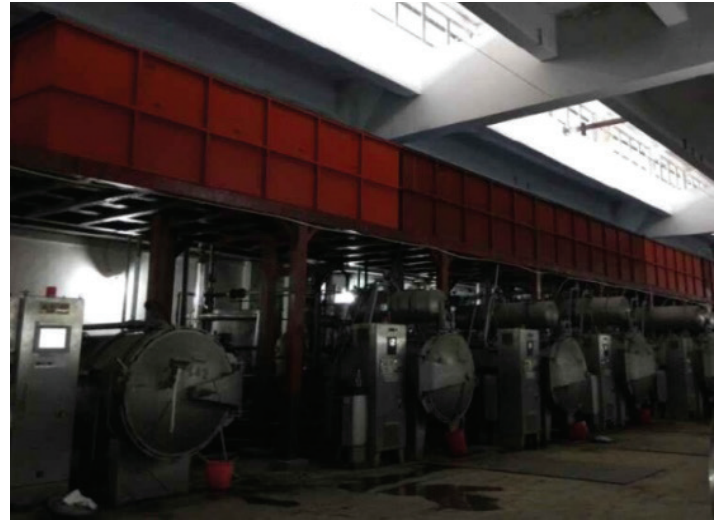
Newly installed cooling water recovery tanks
