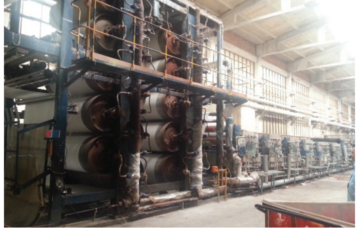
Updated steam trap system for drying cylinders
