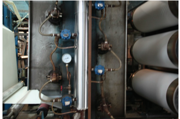
Upgraded steam trap system
