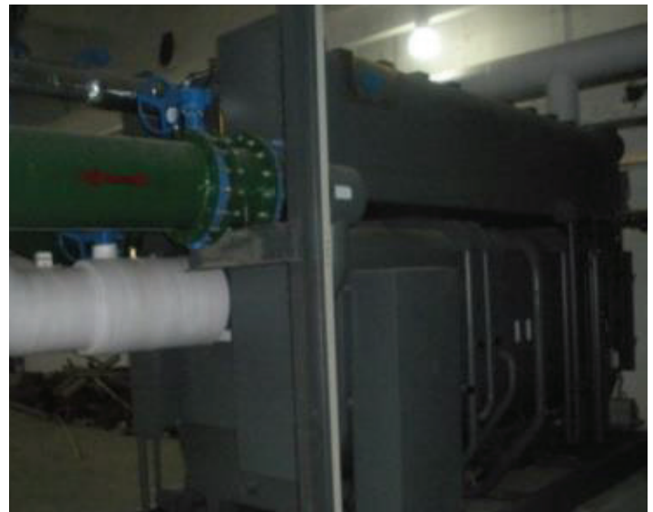
Lithium bromide air conditioner that uses condensate
