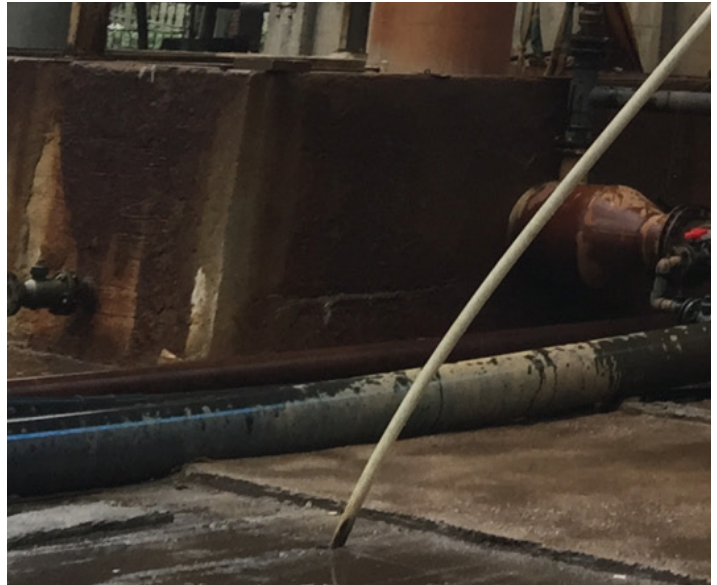
Process water reuse system
