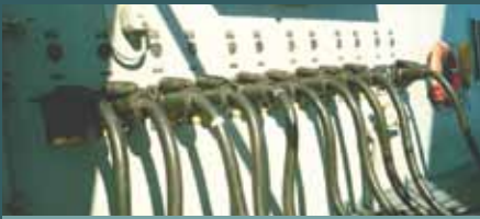
Shore-power connection on a navy ship
