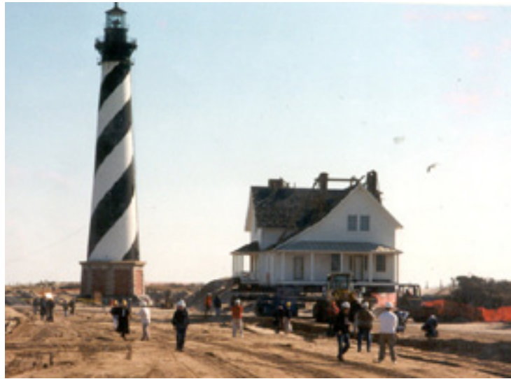
The principal lighthouse keeper’s quarters being moved at Cape Hatteras NS, in advance of the move of the lighthouse itself.
