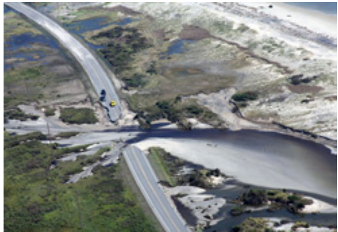
NC Highway 12, Hatteras Island. Photo: FWS.
