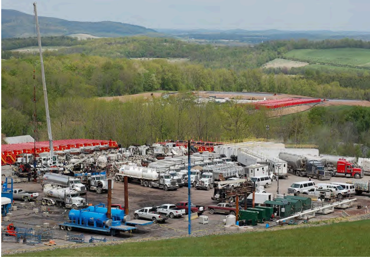
Figure 5. Well site with equipment (and pits in the background) in preparation for hydraulic fracturing in Troy, Pennsylvania. Source: SGEIS, supra, at 5-90.
